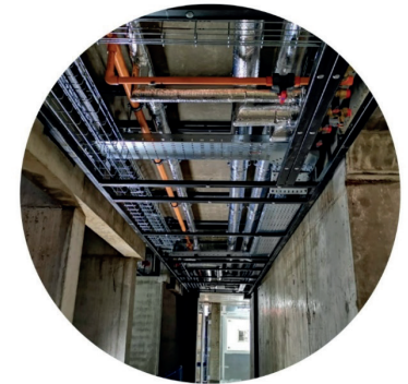
Riser and service
